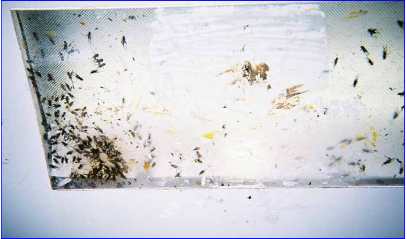
Dead insects trapped in light fixtures (above)
