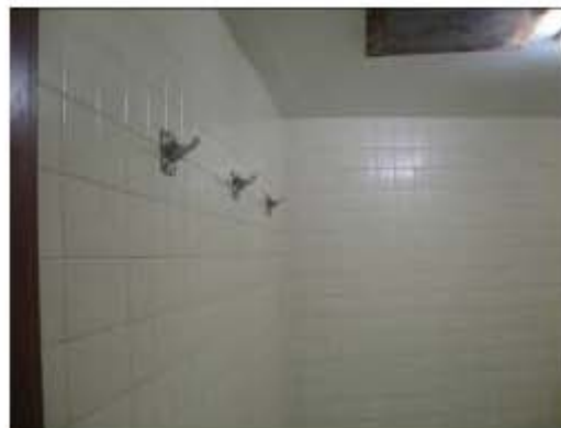
Unsafe Rigid Shower Hooks
