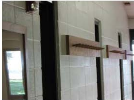
Unsafe Coat Hooks in Dayroom
