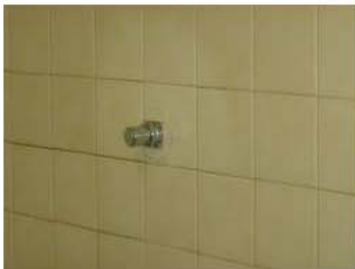
Unsafe Shower Control
