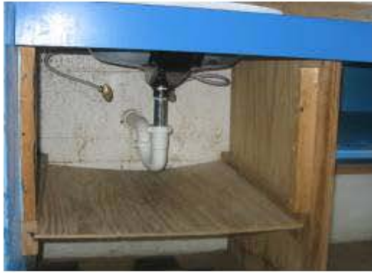
Exposed Unsafe Sink Pipes
