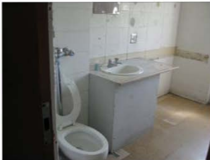
Unsafe Porcelain Toilet and Sink
