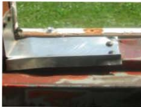
“Repaired” Metal Window Frame
