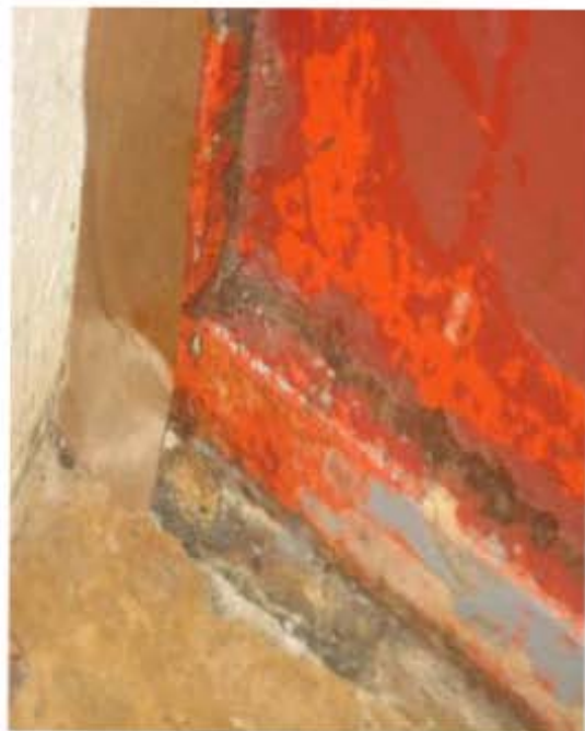
Close-up of Metal Plate
